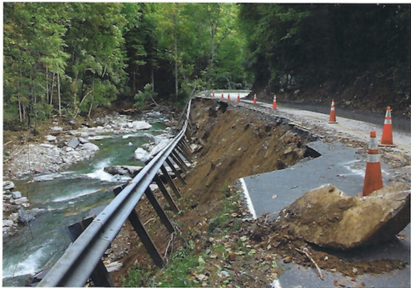
Hurricane Helene washed out roads like this one in Asheville, North Carolina, and caused mudslides and flooding that sent homes floating downriver.
